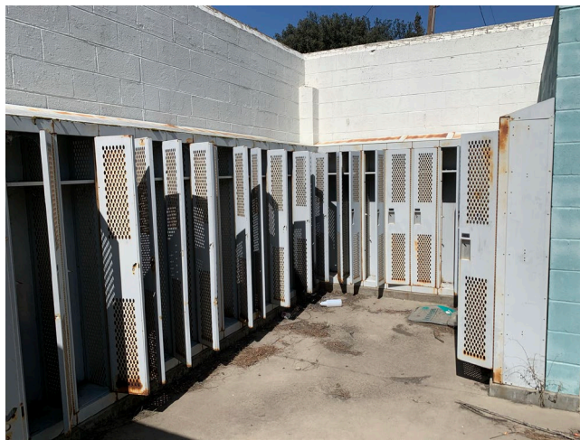
Photo 2 – Bath house locker room non-asbestos-containing concrete and concrete masonry unit (CMU) mortar
