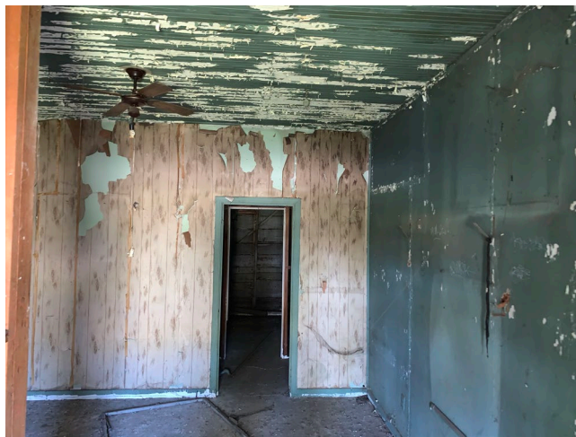
Photo 17 – Park personnel building, deteriorating lead-containing paint on ceiling and walls
